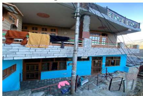
Discontinuity in vertical members over height- Kullu, Himachal Pradesh
