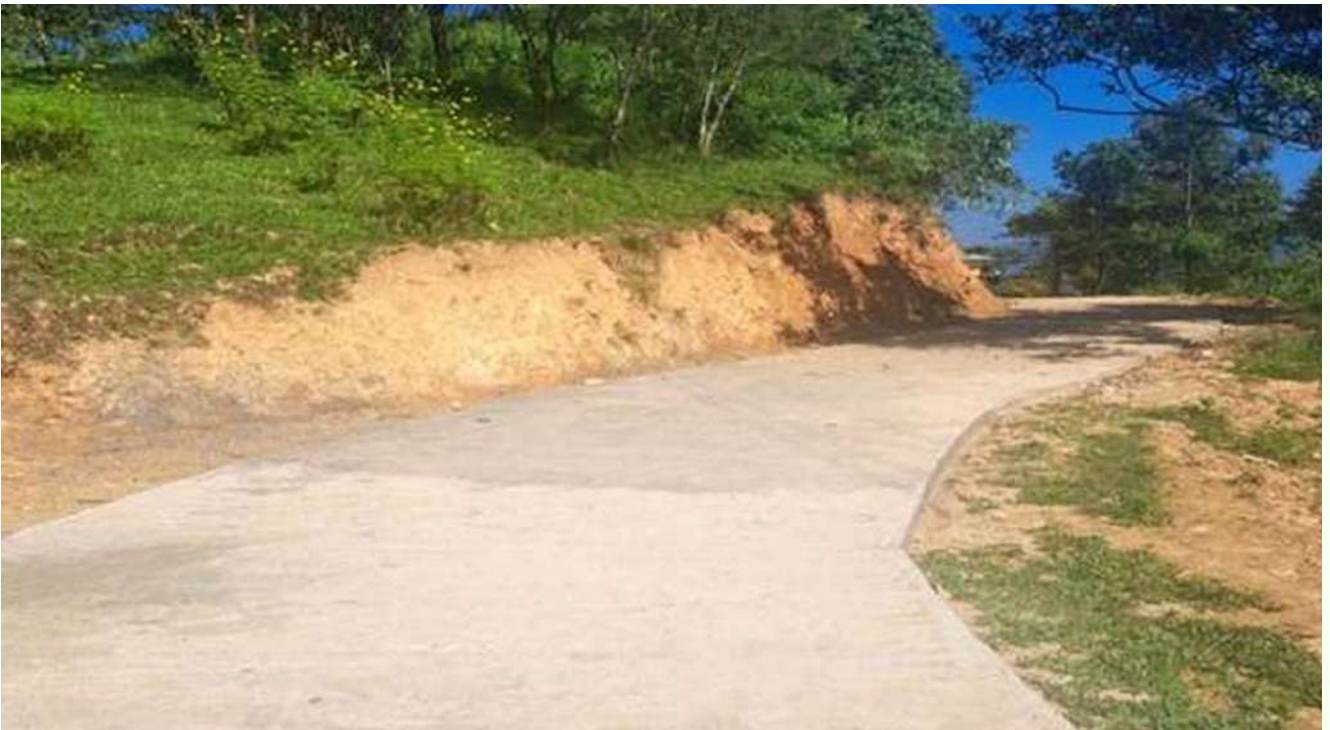
Construction of PCC Pavement from P Vanhne Residence to Sub Centre at Laki Block- Tipa, District - Siaha, Mizoram. Date of completion of work - 15.03.2024 (2023-24).
