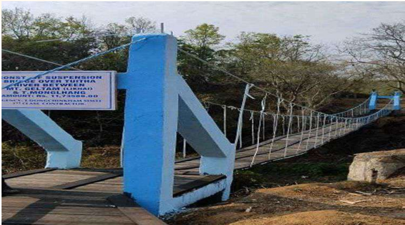
Construction of Suspension Bridge over Tuitha River between M. T Geltam (Likhai) & T. Monglhang, at Likhai, Block- Singhat, District - Chura Chandpur, Manipur. Date of completion of work–11.03.2024 (2023-24).
