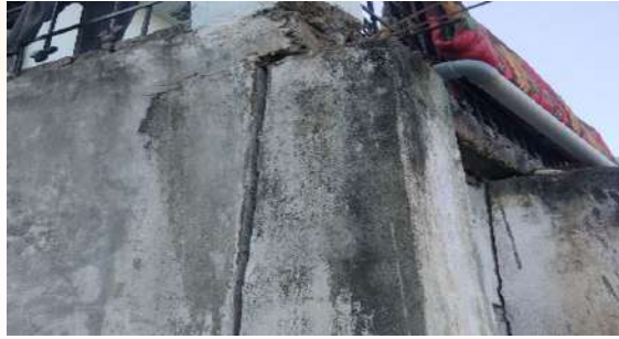
Improper beam-column connection- Pauri, Uttarakhand
