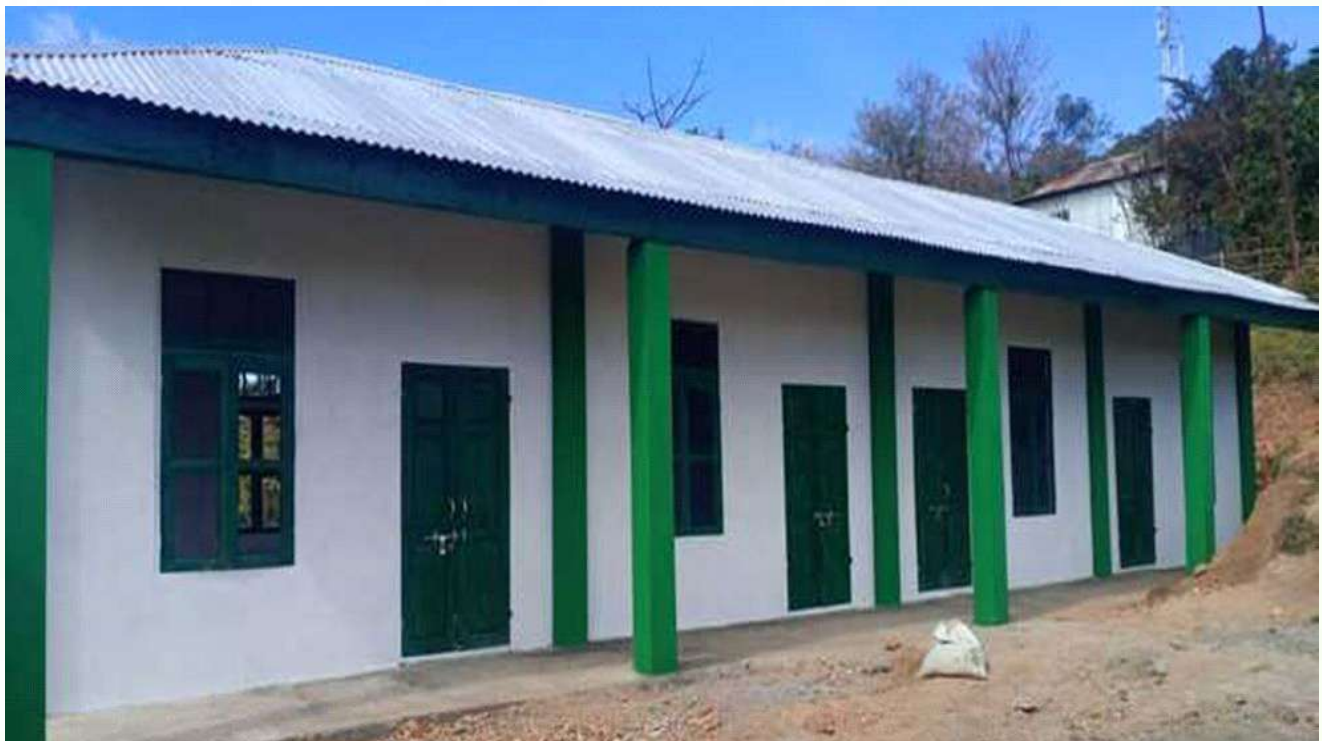
Construction of Govt Middle School at Sentetfiang, Block- Sangau, District – Lawngtlai, Mizoram. Date of completion of work–30.04.2024 (2024-25).
