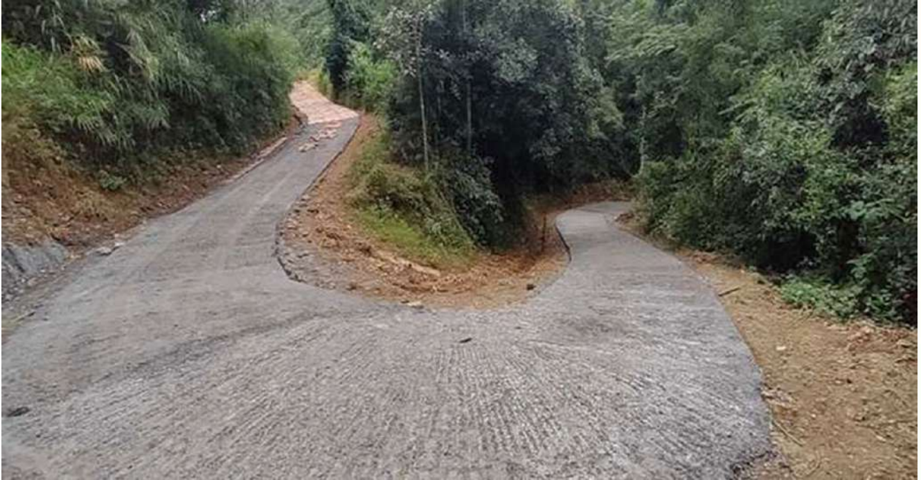
Construction of PCC flooring of jeep road from Lungphunsang to Zokhua at Zokhua, Block & District - Champhai, Mizoram. Date of completion of work - 30.04.2024 (2024-25).
