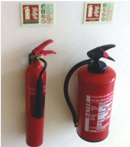
Figure 2.15 CO 2 and water extinguishers and information posters
