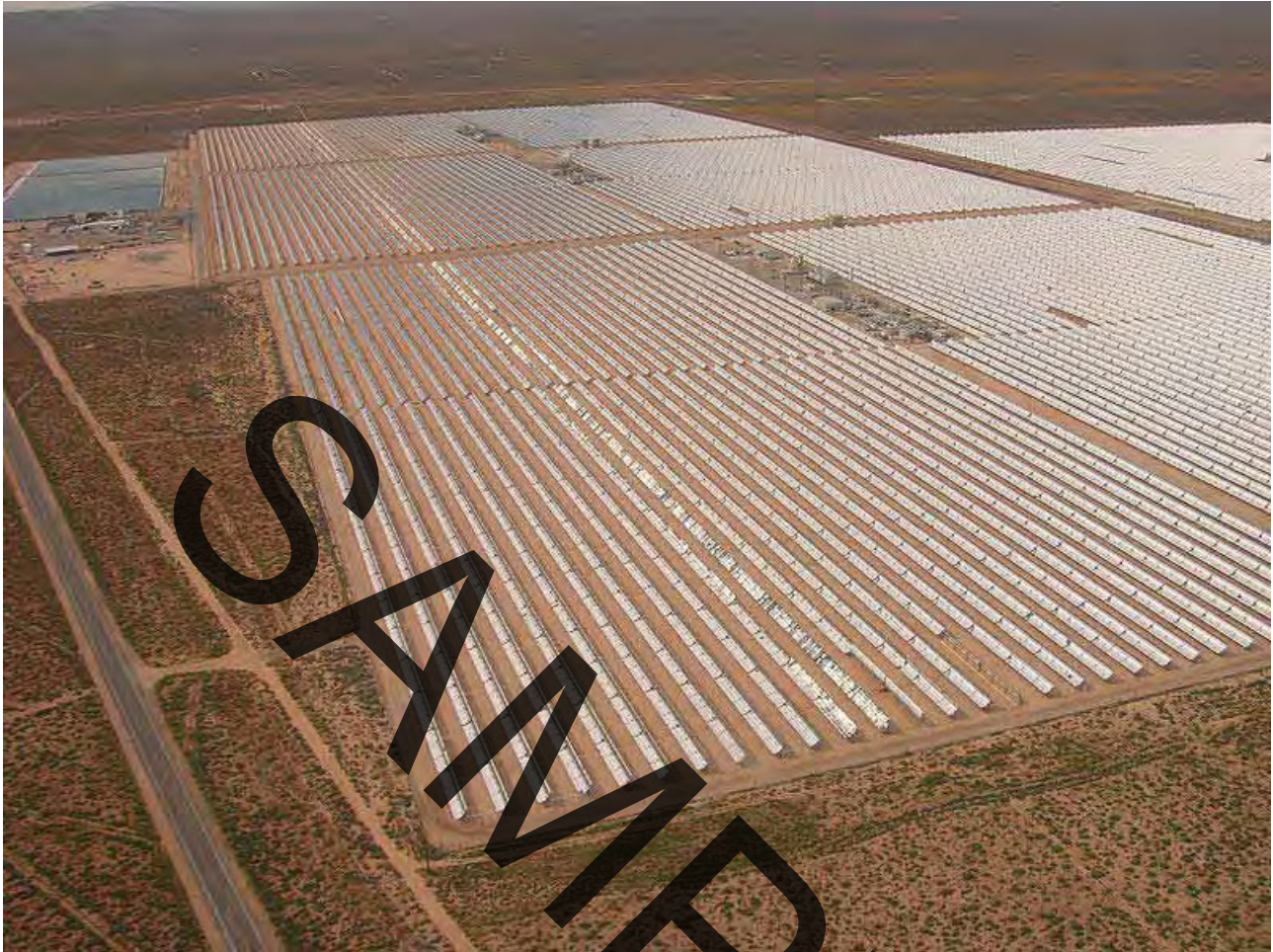
At Nellis Air Force Base in Nevada, 70,000 solar panels are linked together in an array that can generate 15 megawatts of electricity for the base. Photo credit: U.S. Air Force.
